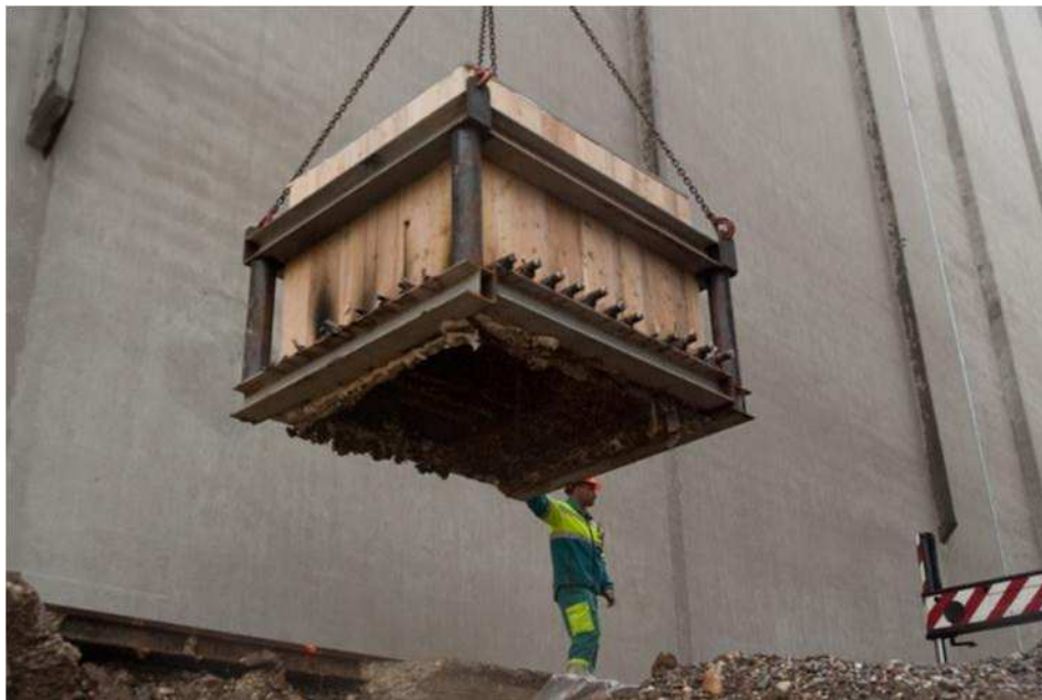
Fig. 10: The site foreman directing the crane operator with the block hanging in the air.
