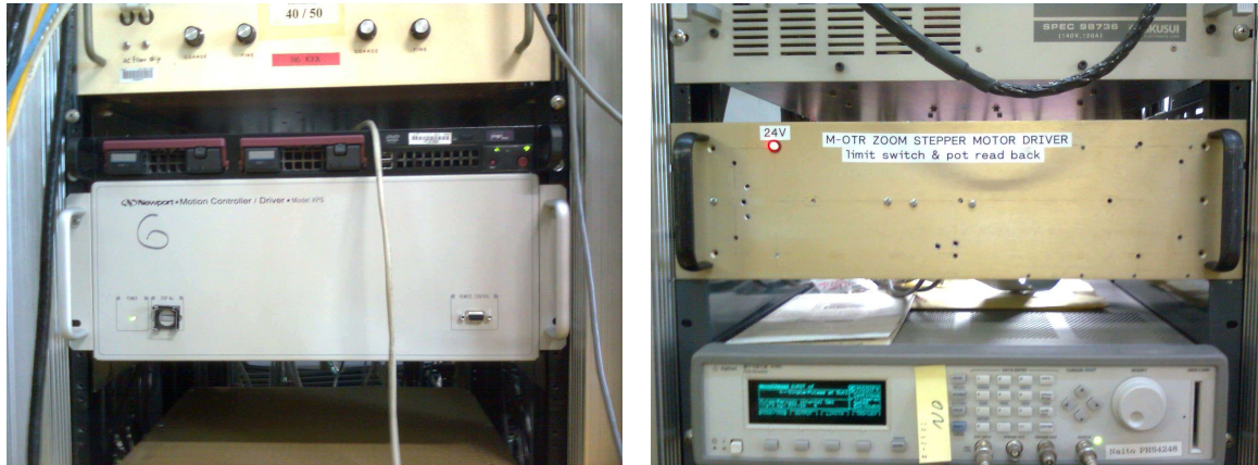
Figure 3.23: Multi-OTR controllers mounted in the racks. In the left the Newport XPS for motion control, in the right the zoom stepper motor driver.
