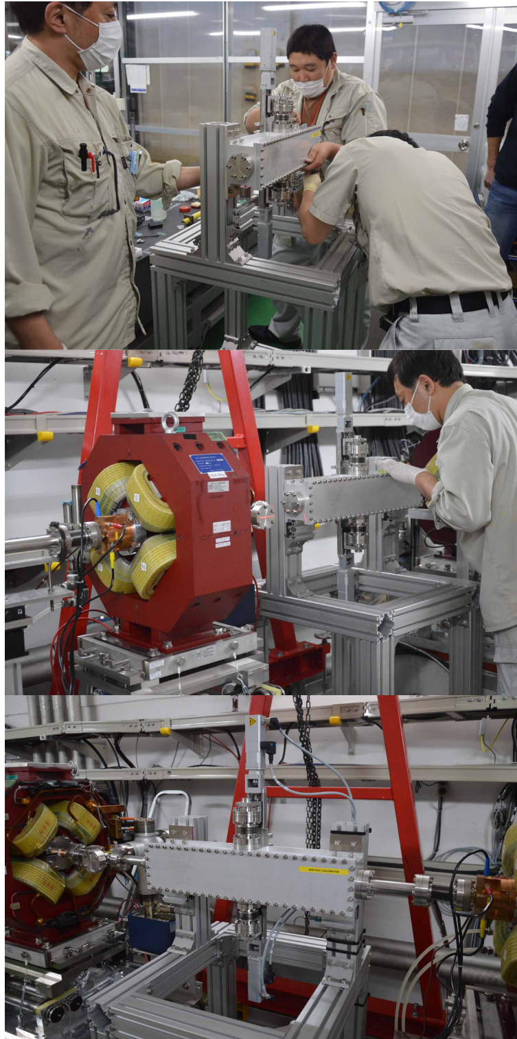
Figure 5.10: Mechanical support fabricated at KEK for the installation of the vertical collimation system into the ATF2 beamline (top). Vertical collimation system installation and alignment procedure (middle). Vertical collimation system after installation in the ATF2 beamline (bottom).
