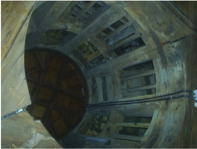
Fig. 258: Royal Palace of Aranjuez, southern tower, view of the central cylinder of the spire
