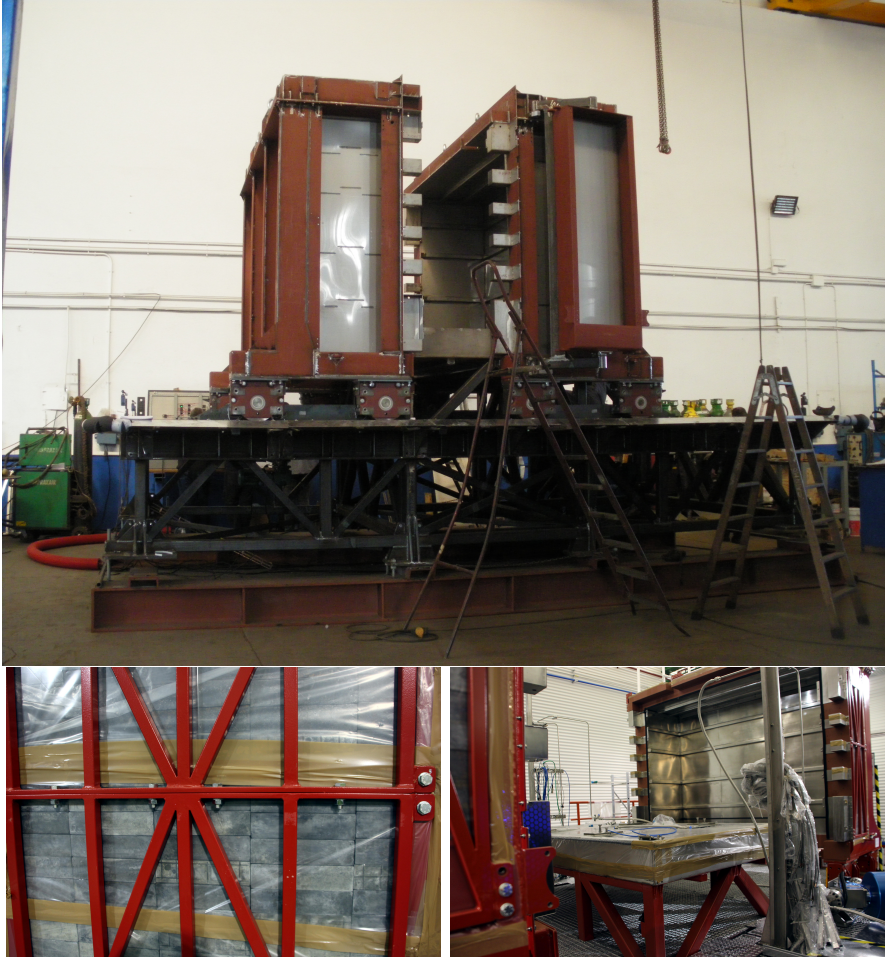
Figure 4.15: Shielding structure during construction prior to any equipment and installation. Lead bricks conforming one wall of the shielding castle. View the shielding castle, without detector fixed on the pedestal, installed at Hall A of the Laboratorio Subterráneo de Canfranc
