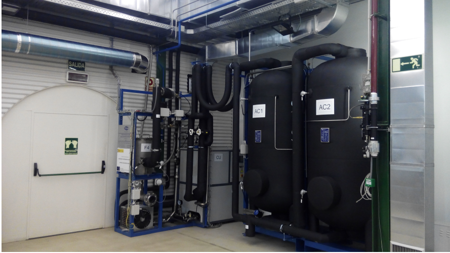
Figure 5.12: Radon abatement system installed at the LSC.
