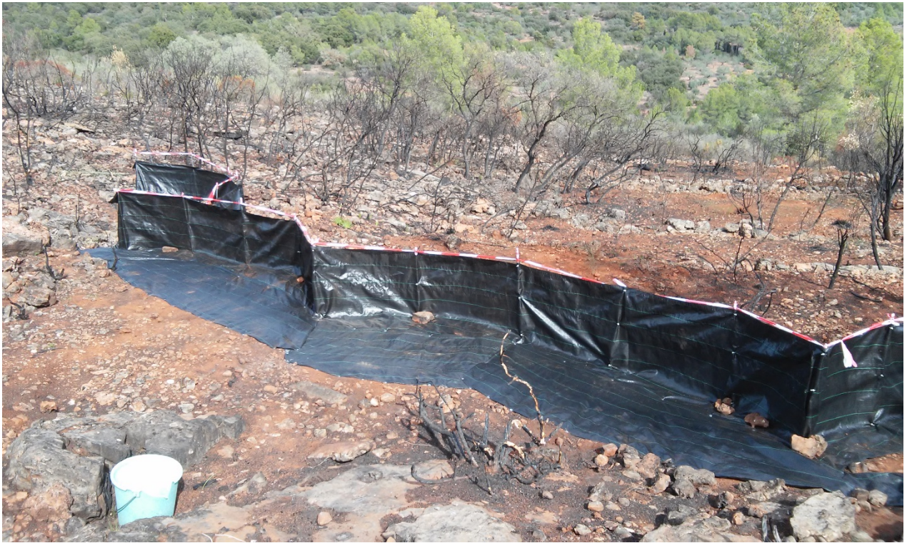
Fig. S3. Sediment fences constructed at the foot of the burned slope.
