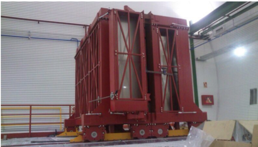
Figure 3.15: Top: Detailed view of NEXT shielding structure in its open position, with NEW vessel placed on the anti-seismic platform. Bottom: View of the shielding structure in its closed position during installation.
