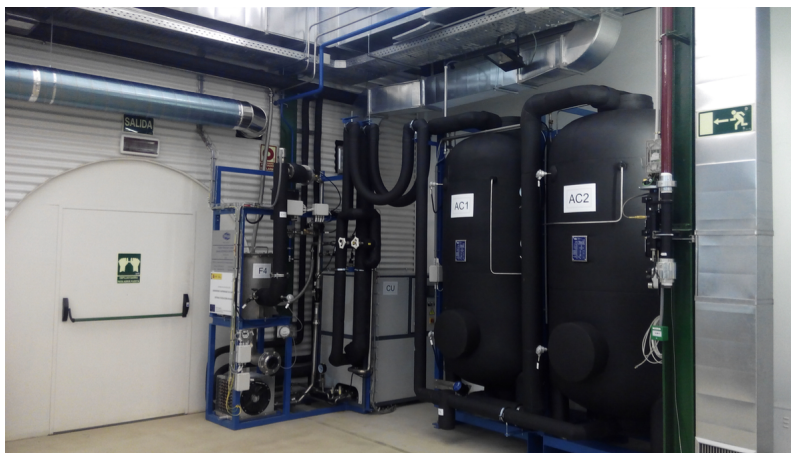
Figure 4.8: Radon Abatement system by ATEKO installed in LSC Hall A.
