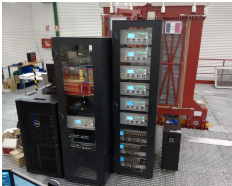
Figure 3.19: NEW electronic racks and the Slow Control PC during installation.
