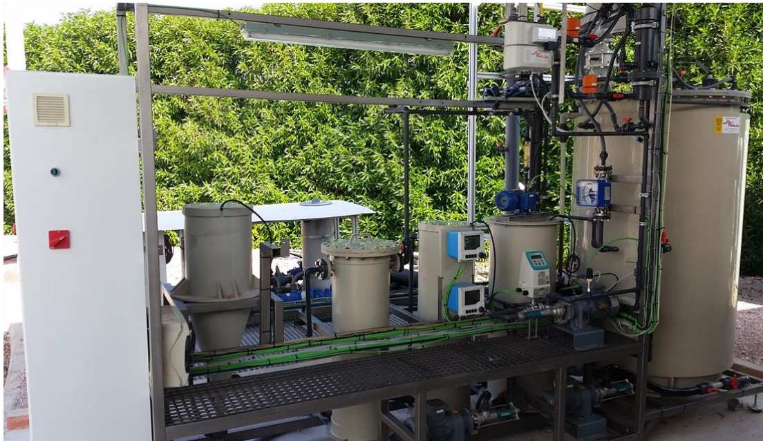
Figure 3.4. Anaerobic co-digestion pilot plant: layout (a) and experimental set-up (b). ET: equalisation tank; AnR: anaerobic reactor; PT: purge tank; MT: membrane tank; DV: degasification vessel; CIP: Clean in Place tank; BGM: biogas meter.
