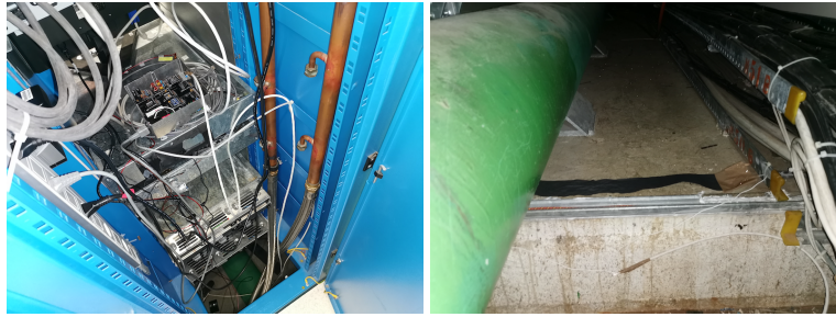
Figure 6.27: Reliance box (left) monitoring the Smart Paper (right) in the entrance of the tunnel between USA15 and the CV room.
