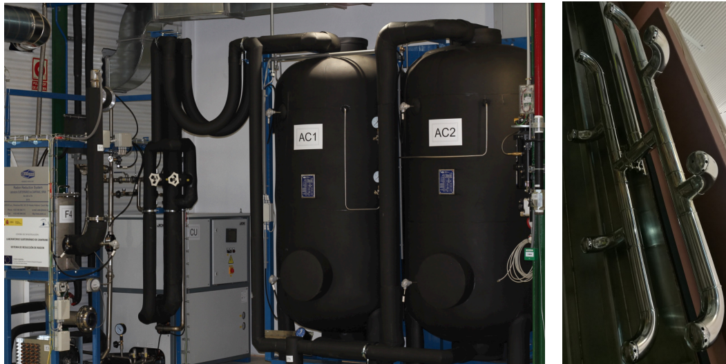
Figure 7.2.: Radon abatement system by ATEKO installed in Hall A of the LSC (left) and detail of the pipes supplying the radon-free air inside the outer castle (right).
