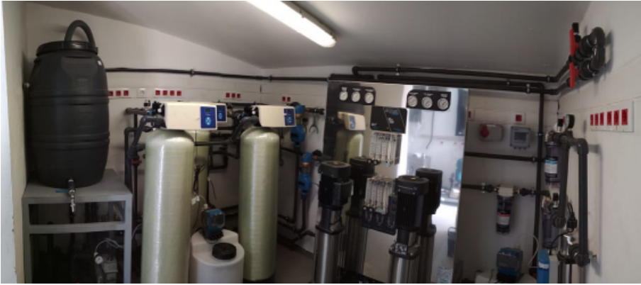
Figure B.5 – Picture of the water purification system.
