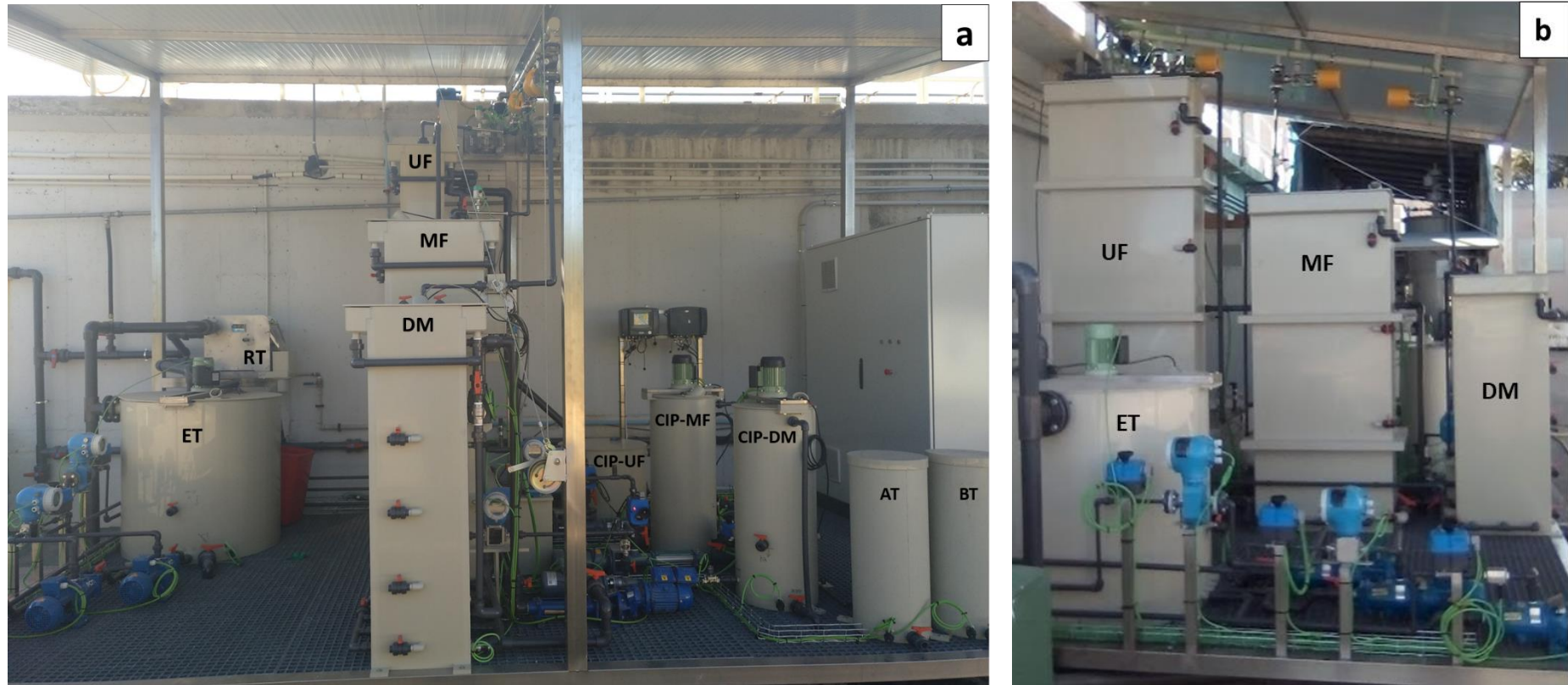
Figure. 3.2. Complete picture of the membrane pilot plant: (a) side face and (b) frontal face.
